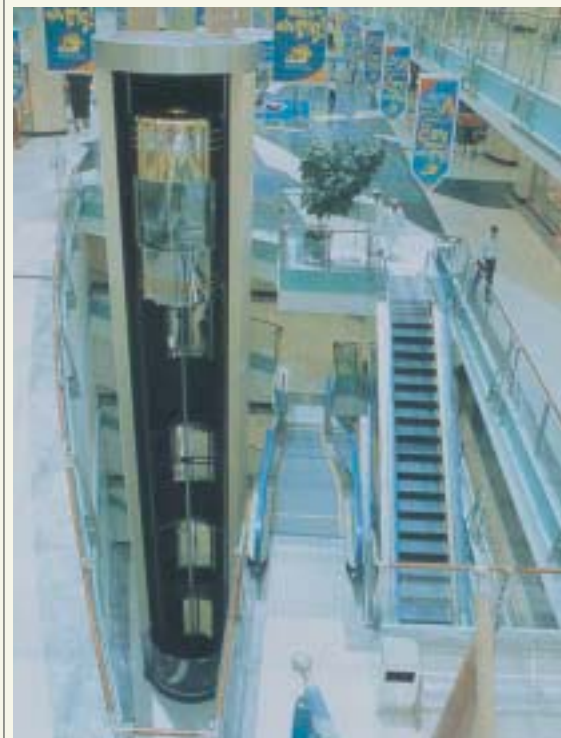
Observation elevators and escalators serve the shopping mall
